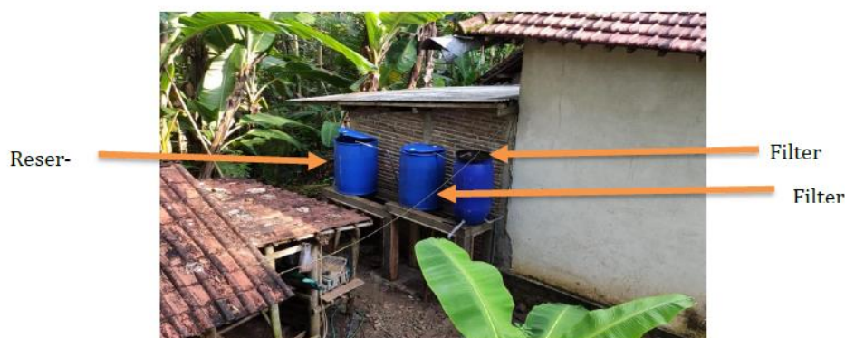
Figure 2. The results of the installation of the filtration system are clean water treatment technology.
